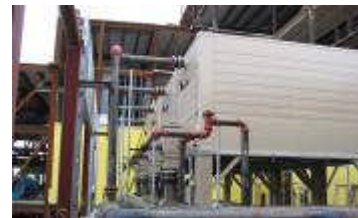
Combined Heat and Power
